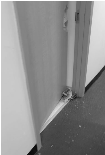
Door handles were broken off.
